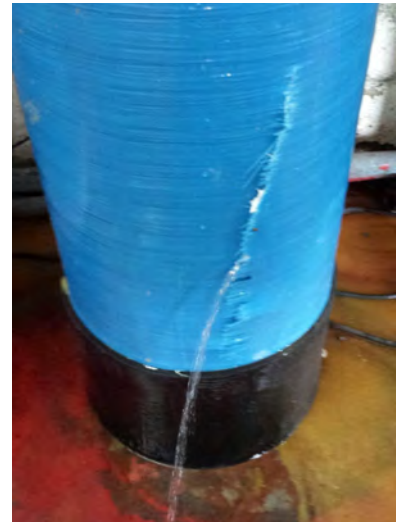
4. Broken Fiber and Inner Polyethylene Shell Negative Pressure caused by siphon and Pressure Pump (RO) after filtration media tank. No Vacuum Breaker installed.
