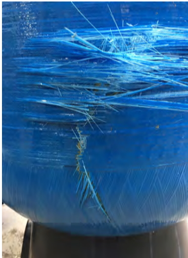
2. Implosion Tank - Broken Fiber Negative Pressure caused by siphon and Pressure Pump (RO) after filtration media tank. No Vacuum Breaker installed. Polyethylene inner shell damaged.
